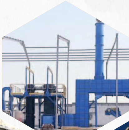
ADVANCE INCINERATION SYSTEM WITH FLUG GAS TREATMENT
